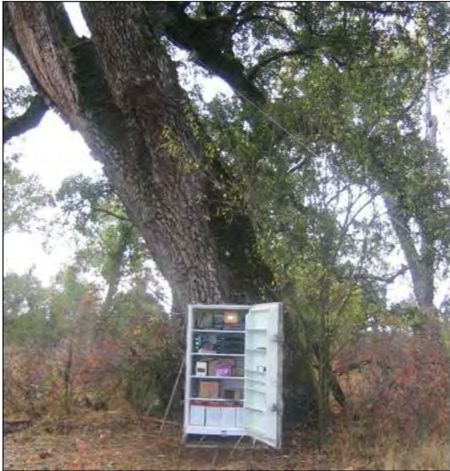
Figure 7. The modified refrigerator contains the DVR's, power controls, equipment and storage boxes, monitor and batteries. The cable above the lock box is the anchoring cable to the two main cables suspending the camera over the creek.
