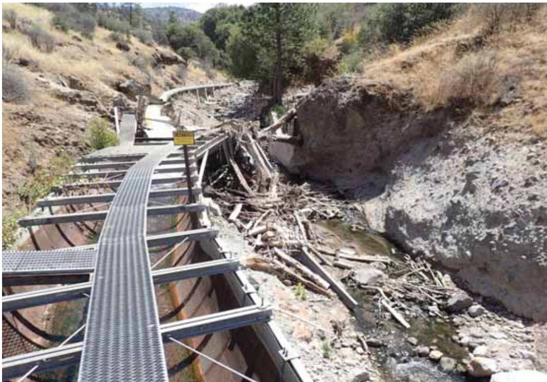
Figure 8: Photograph of Soap Creek Canal and debris associated with riparian vegetation loss in the area. Difference in elevation between walkway atop canal and stream bed is approximately 15 ft.
